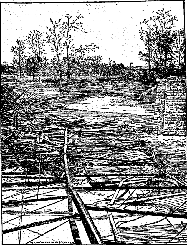
Tornado near Connersville, Ind., May 14, 1883, about 7:00 P. M. - Ruins of an iron bridge lifted from abutments and dashed into the river below. From a Photograph.
